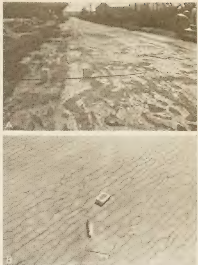
FIGURE 11.—INADEQUATE DRAINAGE CONTRIBUTED TO BASE FAILURE ON THESE EXPERIMENTAL SECTIONS. A, BOTH BASE AND SURFACE FAILED ON EXPERIMENT 2, SECTIONS C AND D. SAND WAS USED WITH A COLD-APPLICATION MATERIAL FOR SURFACE TREATMENT, RESULTING IN A RICH, PLASTIC MIXTURE. B, BADLY CRACKED AREA ON EXPERIMENT 3, CAUSED BY A PLASTIC SUBGRADE.
